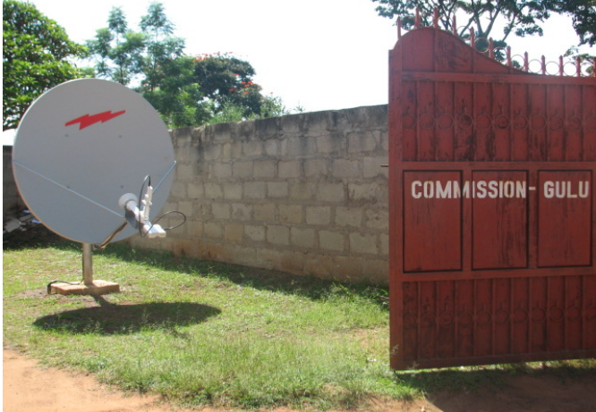
VSAT Communication device installed at AC-DRT Gulu [IOM photo]
